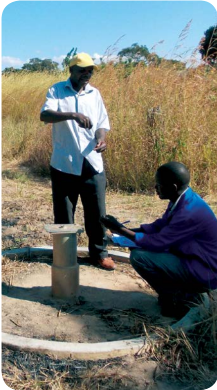
Borehole abandoned due to dropped-in pipes, Mpika, Zambia
